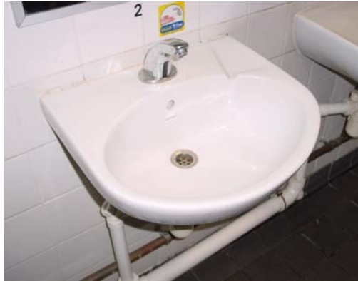
BM administration building 3/F male toilet
