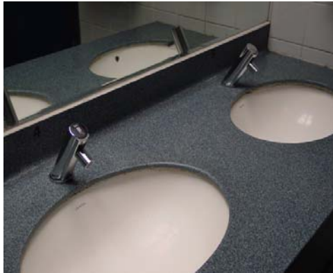
BM administration building 4/F male toilet
